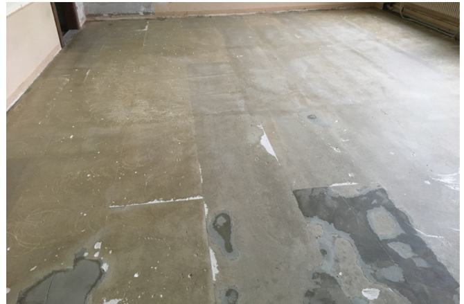
Existing substrate that needs refurbishment
